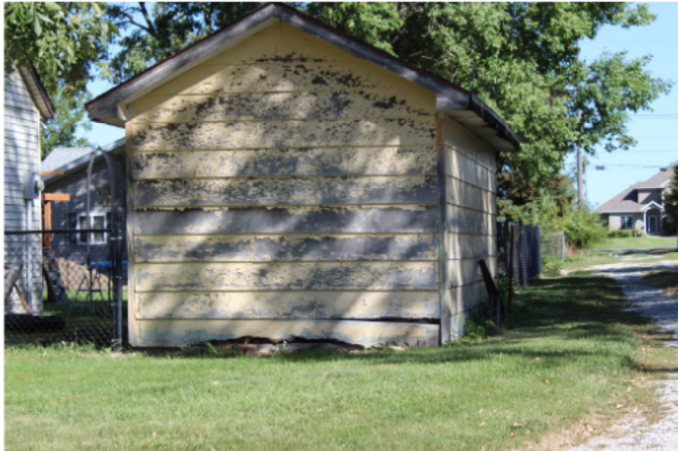
Photo 1: Structure in Poor Condition
