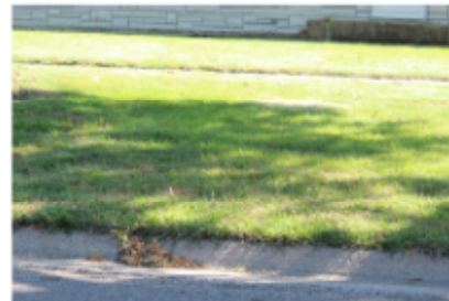
Photo 5: Vegetation gathering due to poor drainage in gutter
