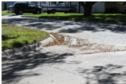
Photo 2: Poor drainage in gutter
